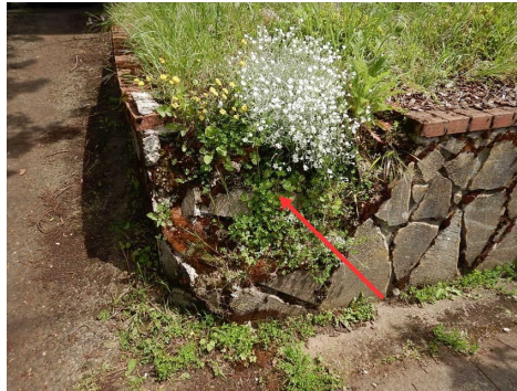
Damage at wall
