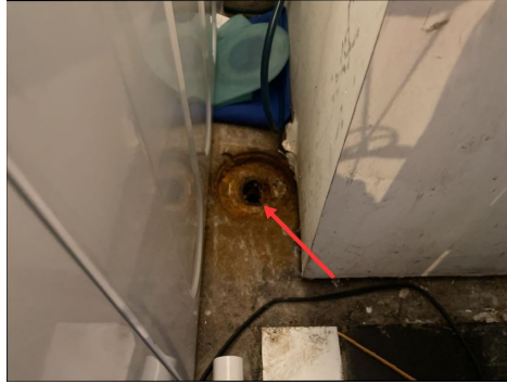
Stains at floor drain
