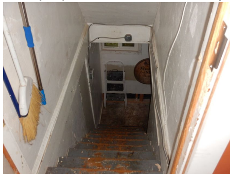
No railing present
