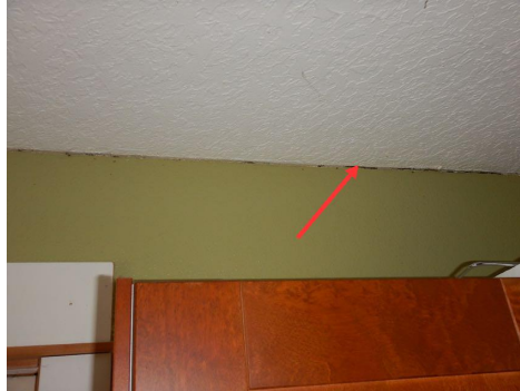
Cracks at walls
