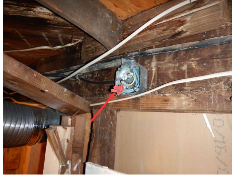
Missing box cover
