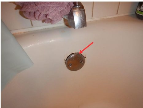
Rust at tub
