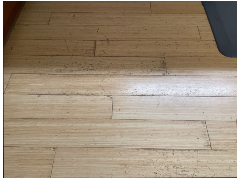
Heavy wear at floor
