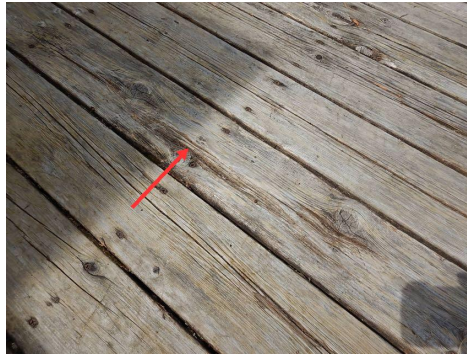
Rot at deck
