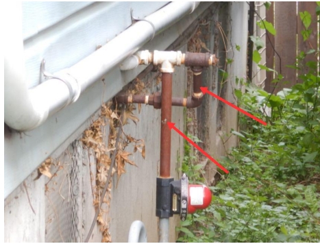
Pipes not protected
